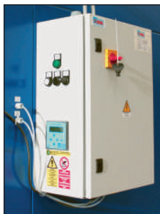
ELECTRIC CONTROL BOARD
